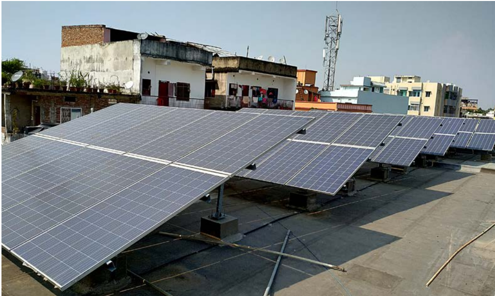
Generation of clean energy through rooftop solar projects in Bhagalpur
