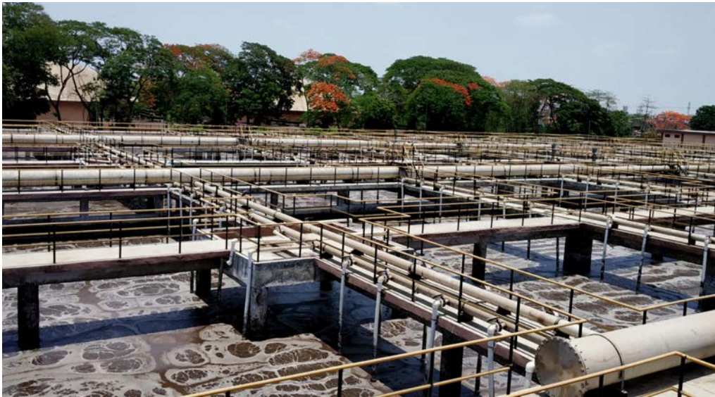
Anjana STP at Surat retrofitted with SCADA & energy generation capabilities
