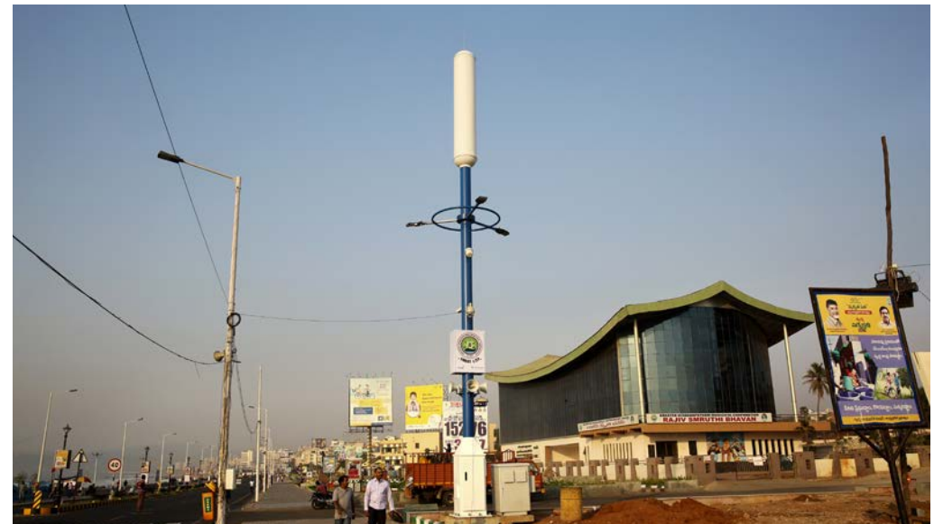
Visakhapatnam Smart Poles
