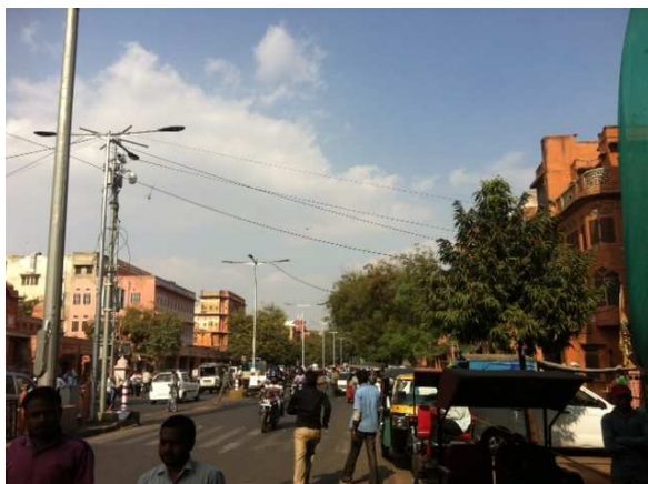
Overhead cables, broadband ,highmast pole
