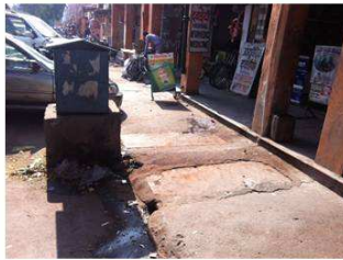
JUNCTION BOXES/ FEEDER PILLAR
