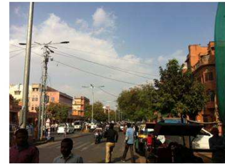
OVERHEAD CABLES, BROADBAND, HIGHMAST POLE
