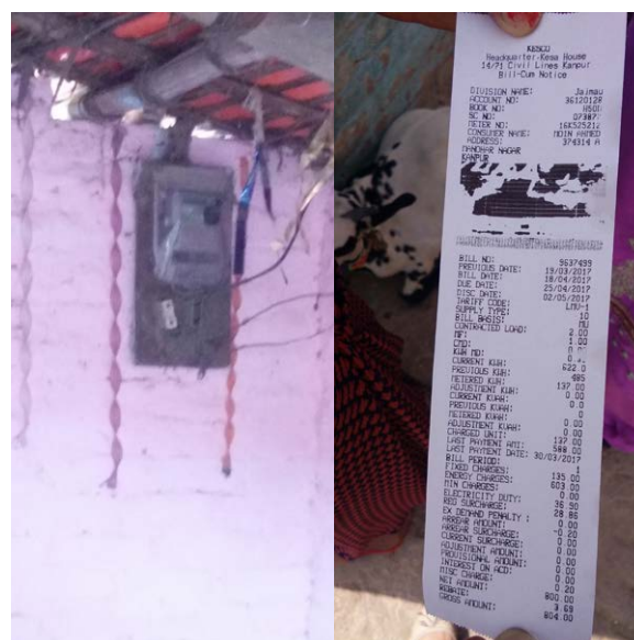
Figure 7 Electricity meter and bill for power charges for water supply in Manohar Nagar
