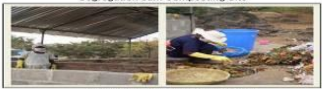
Segregation cum Composting Site Secondary Segregation of collected waste
