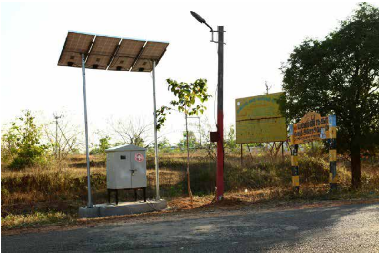
FIGURE 10: Solar street lighting
