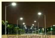
Smart Street Lighting (LED)
