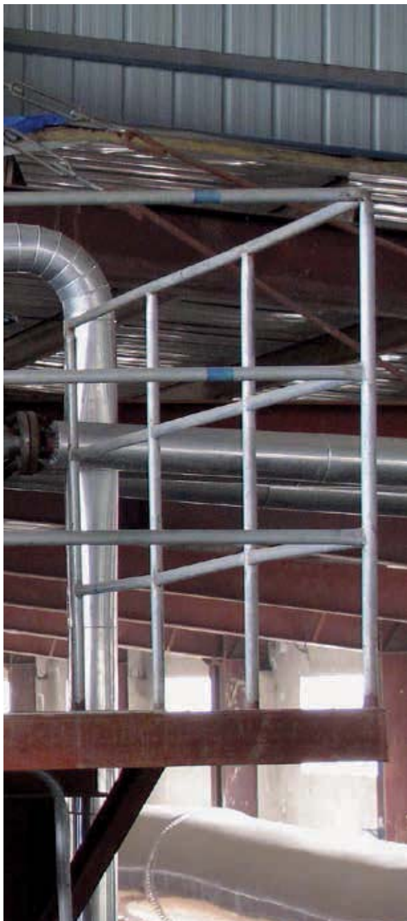
Part of the Coal-Gangue Brick Waste Heat Recovery Power Generation (WHRPG) boiler at Xinrong pilot plant ©The China Climate Change Partnership Framework (CCCCPF)/China Joint Programme
