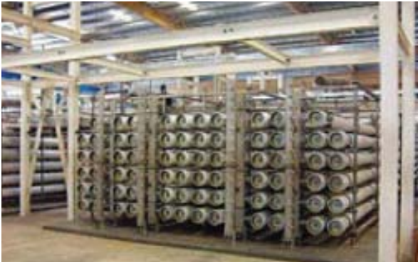
The plant has a total ultrafiltration (UF) membrane area of 304,640 m 2 arranged in 68 skids. (Source: IWA)
