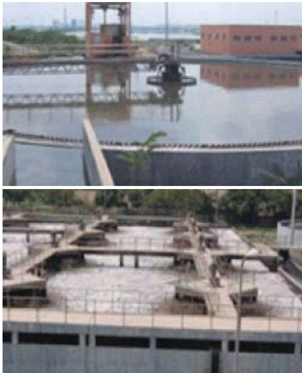
Wastewater treatment plant (Source: IWA)
