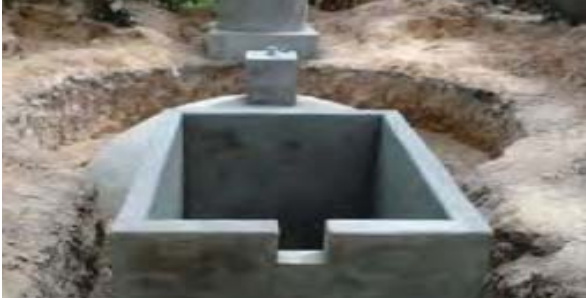
A nearly completed biogas digester, showing the mixing tank (rear), biogas chamber (middle), and outlet (front). (Source: National Biogas Program, 2011)
