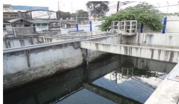
Sequential batch reactor (Congressional STP) (Source: M. Ebarvia)
