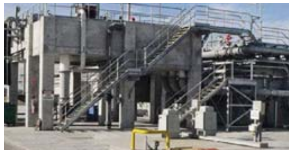
Altona wastewater treatment plant (Source: M. Gieseemann)
