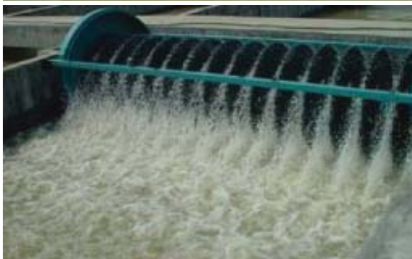
Xiang'an Sewage Treatment Plant (Source: Zhou Qiulin)
