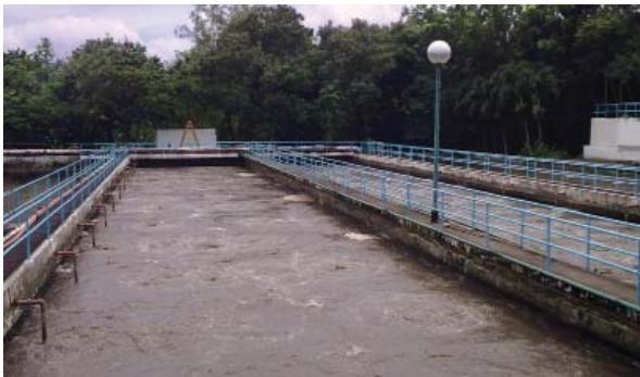
Activated sludge with extended aeration (Ayala Alabang STP) (Source: M. Ebarvia)
