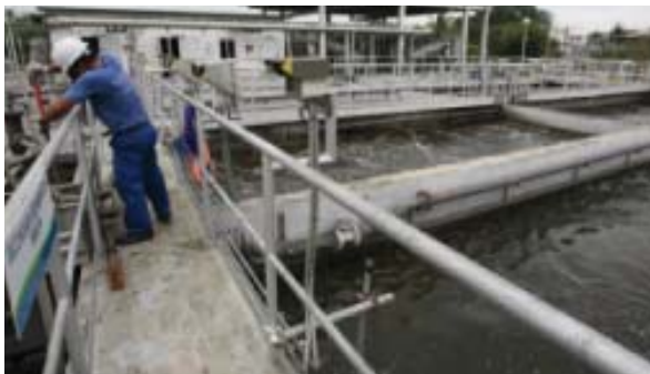
South Septage Treatment Plant (Source: S. Griffiths)
