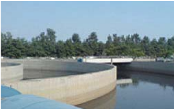
Wastewater treatment plant in Hebei (Source: ADB)
