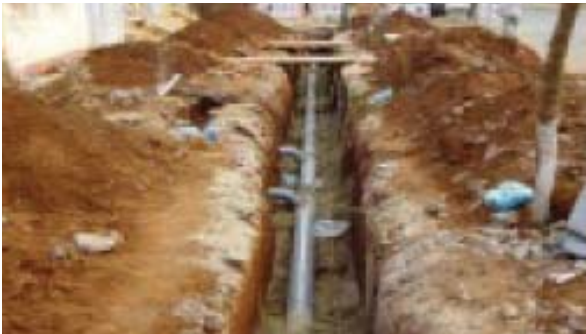
Sewerage system (Source: Viet Anh Nguyen)
