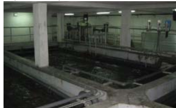
Pineda STP (Pasig City): aeration tanks under a basketball court (Source: Steve Griffiths)
