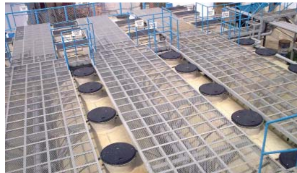
Moving bed biofilm reactor in Johkasou tanks (Paco STP) (Source: M. Ebarvia)
