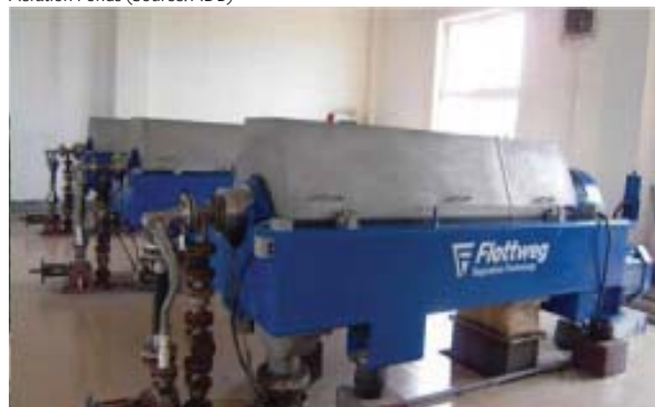
Sludge-Dewatering Centrifuges (Source: ADB)
