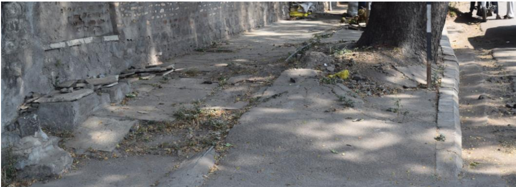
Figure 5 Irregular levels across footpaths
