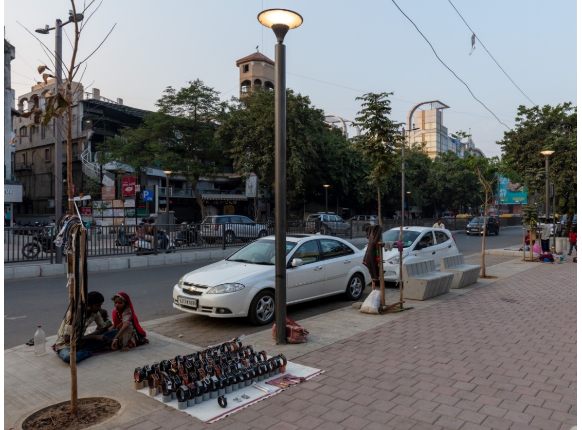
Installed Light Poles
