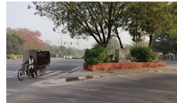
Figure 32. 06 poor quality refuge islands, paint markings unclear reducing road safety greatly. The intersection has good green cover providing a shaded experience to pedestrians and cyclists.
