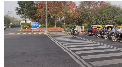
Figure 23. Refuge area is not protected. Road markings are not as per standards. Stop lines not seen, lack of signage.
