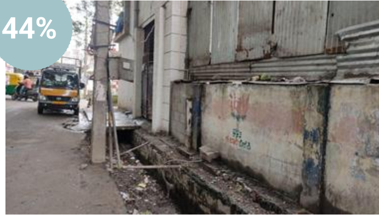
Open drains / Dumping
