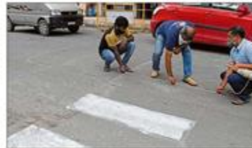
Locals mark a zebra crossing on Siddaiah Road to facilitate safe pedestrian movement. DH PHOTO/SK DHNESH
