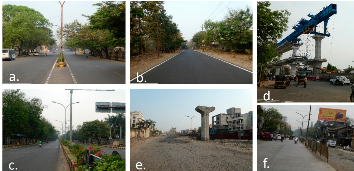
Figure 16. Roads of Nagpur city. (a–c) Avenue plantation along the major roads; (d,e) metro construction work in progress leading to cutting and compensatory plantation of many road side trees; (f) cement road construction projects leaving stressed vegetation along its course.
